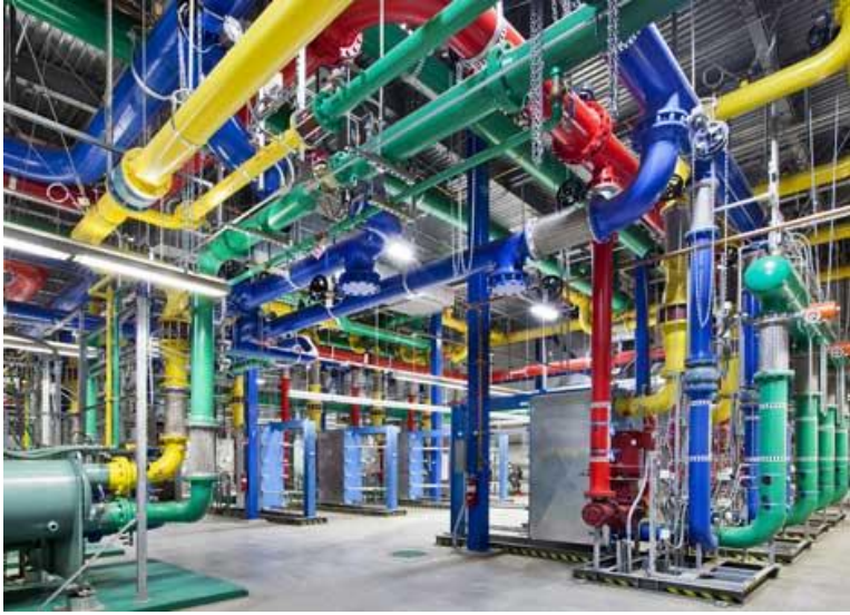
Cooling plant at a Google DC in Oregon
